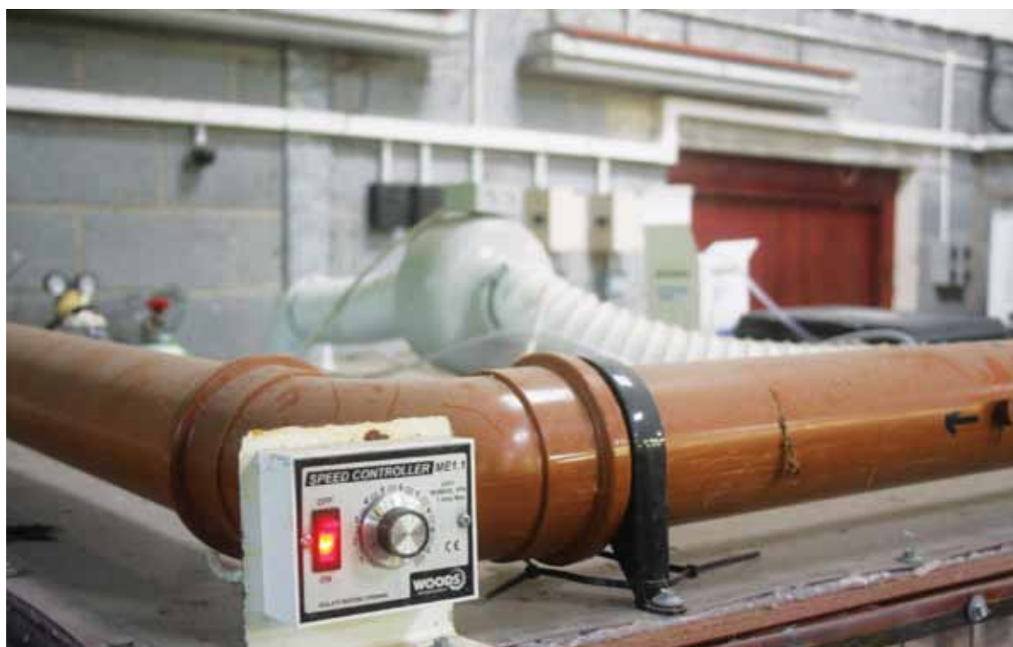
Plate 8: The variable fan speed controller and the inline fan positioned on the top of each chamber, at Aberystwyth University.
