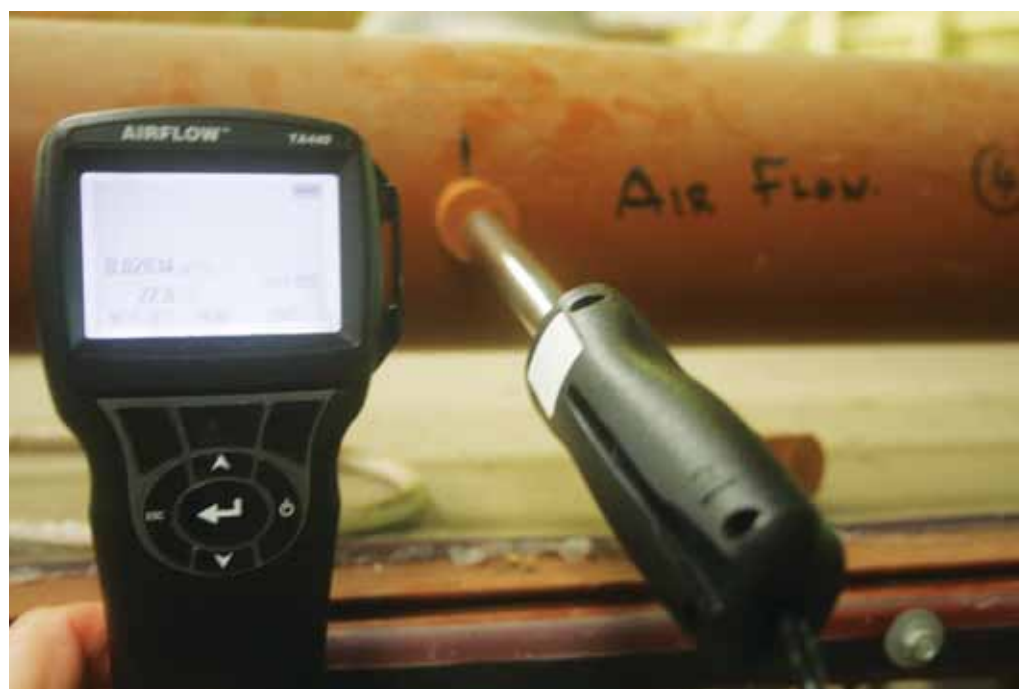
Plate 6: Top of the chamber at Aberystwyth University showing hand held flow meter inserted into the exhaust pipe.
