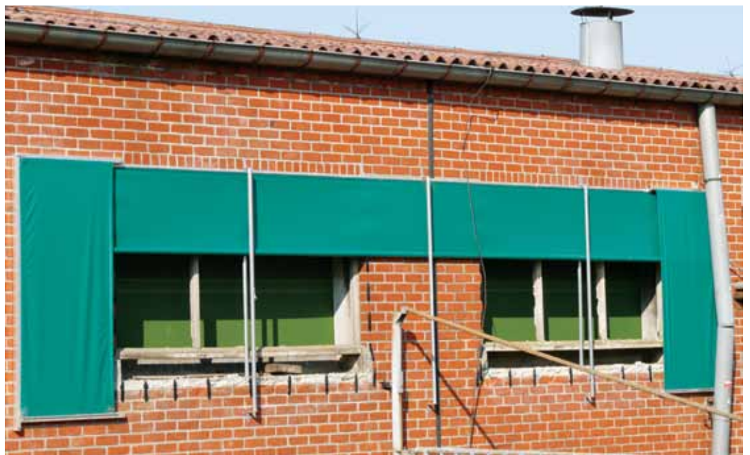
Plate 3: Openings for air inlet, equipped with a fixed wind-breaking net with a porosity of 30% on the inside and an adjustable tarpaulin on the outside.
